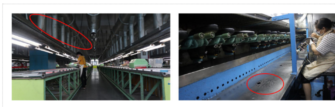
Figure 5: Local exhaust ventilation and use of local fume arm (Photo Courtesy: Nike, Inc.)
