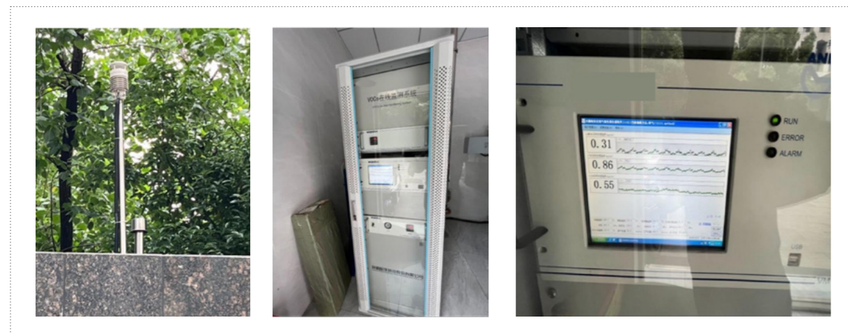
Figure 10: Continuous VOC monitoring system (Photo courtesy: Hefei Ketian Waterborne Science and Technology Co. Ltd.)
